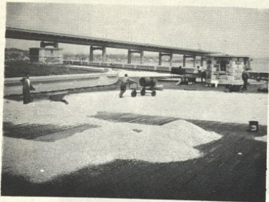
The pictures shown give a good indication of the amount of work and construction that's been going on during the past year. The large parking facilities and two tennis courts were completed just prior to graduation. The entire roof of the fort is being re-tarred and graveled.
