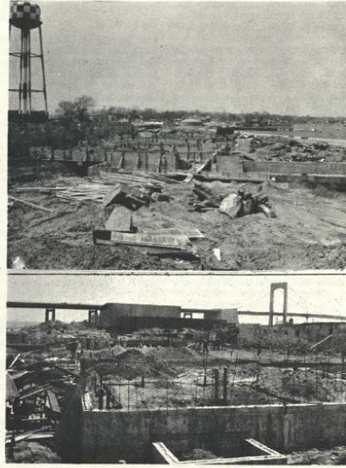
Above - Two views of the present progress on the Science and Engineering building foundations.
