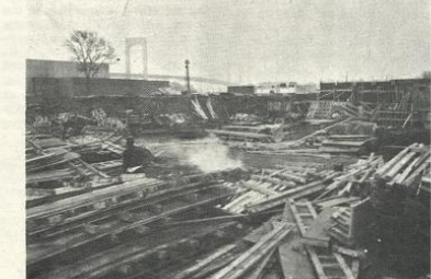
Recent picture of the construction progress on the new Science and Engineering building. photo by Merkel
